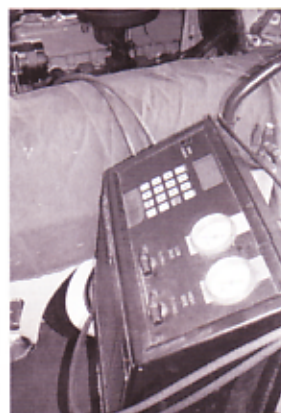
17. Finally, after making sure that all fittings were tight, the system was charged and checked again for leaks.
